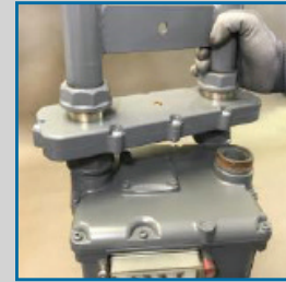
4. Connect the inlet side of the new meter & install a nut plug in the outlet
