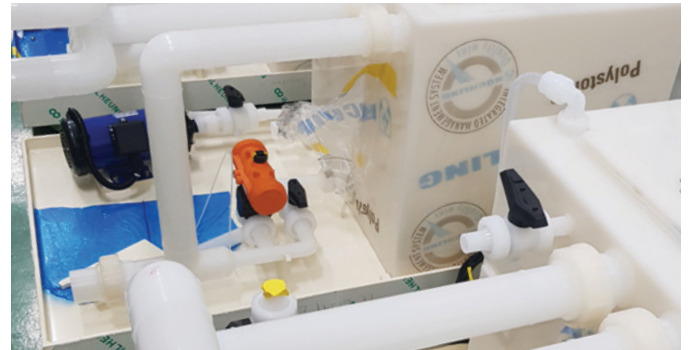
The SYGEF Plus PVDF-HP piping system at ASE Co. Ltd.
