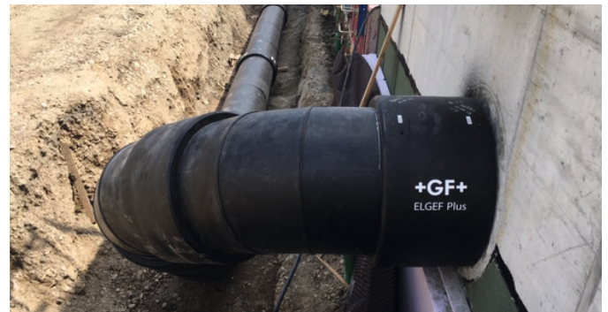
Tight bend of the fresh air duct d710 mm directly on the building.
