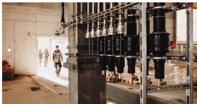
Connection manifold on production machines.
