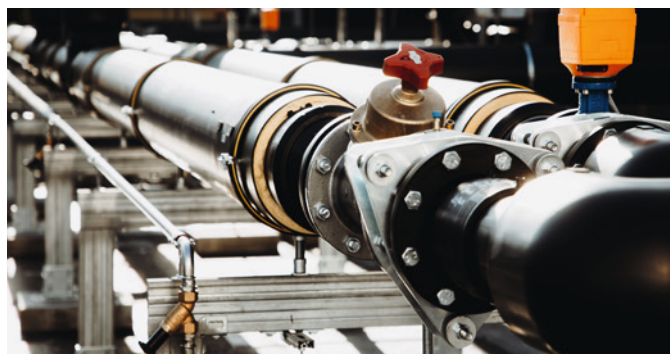
Recooling on the roof of the production hall.
