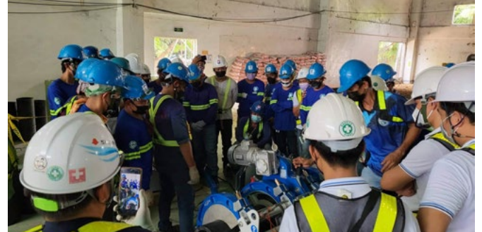
On site training for a safe, fast, and reliable installation of the mission-critical cooling loop.
