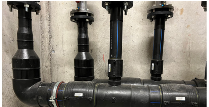
ELGEF Plus is part of a heating system for the Masoala Rainforest – the largest of its kind in Europe.
