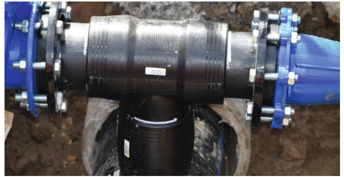
The old fiber cement pipes are relined with a modern polyethylene system. Only small trenches are required to attach lateral outlets.
