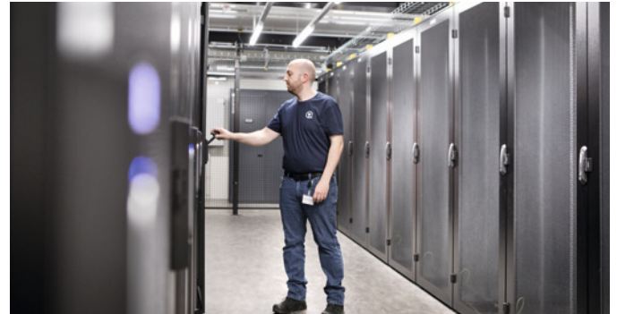
The servers, storage systems and network components in computer centers get extremely hot – cooling is an indispensable process.
