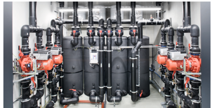
COOL-FIT 4.0 in the BADEN CLOUD® cooling system at the Appenweier site.
