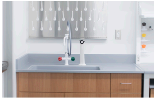
AquaTap™ recirculating laboratory faucets installed in combination with Inline Flow Diverters (IFD) eliminate dead-legs at all points of use to maintain purity throughout the DI water loop.
