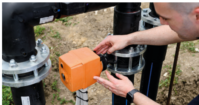
Thanks to electrically actuated valves, the irrigation system has a better response time and can be controlled centrally.
