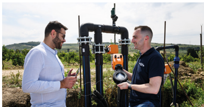
The irrigation system needs to meet high demands – the orange farm covers an area of 50 hectares.
