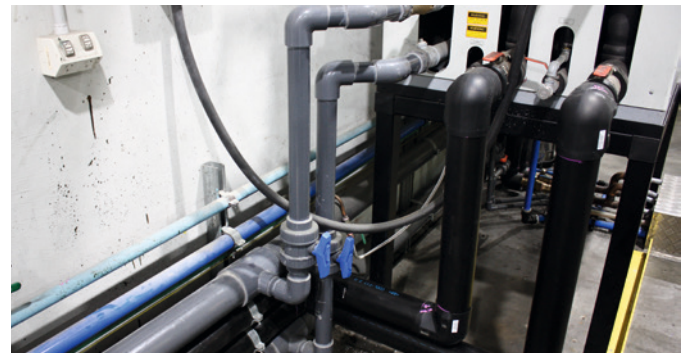
COOL-FIT 2.0 pipes, fittings and ball valves in d63 were installed. PE/SS union adaptors were used to allow flexibility to move the machines.
