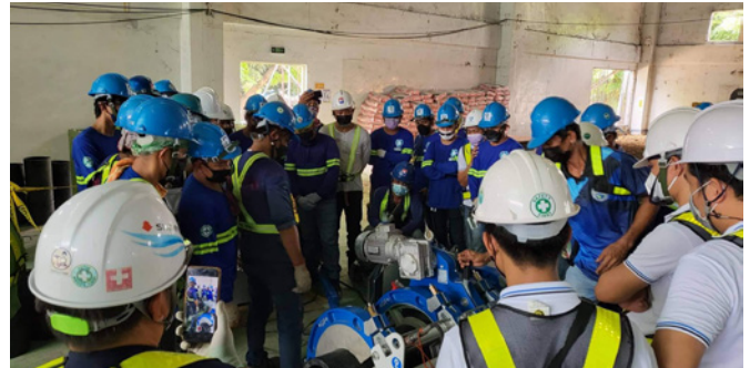
On site training for a safe, fast, and reliable installation of the mission-critical cooling loop.
