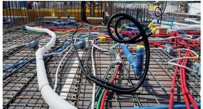
The iFIT pipes (black) are fitted for the drinking water supply to the apartments.
