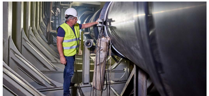
Completed in 2,000 hours by 14 skilled installers, the Oden retrofit overcame tight spaces and system complexity, offering a cost-efficient alternative to metal.
