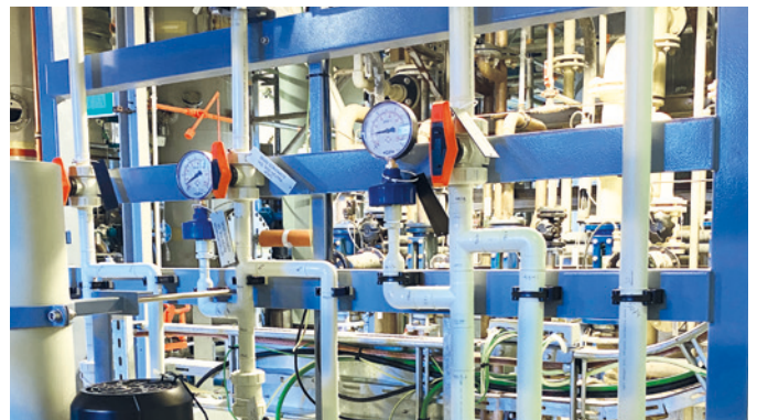
Gauge guards mounted at the end of the piping system.
