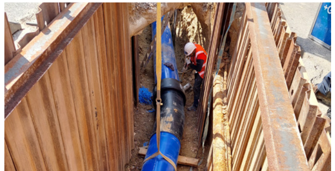
In order to ensure a fast and simple installation, the utility decides to reline the old cement pipes.
