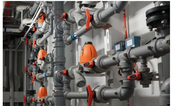
The corrosion- and maintenance-free polybutene system INSTAFLEX provides operational safety to Seabourn Pursuit. Source: GF Piping Systems
