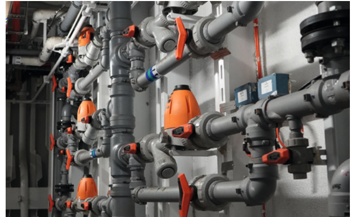
The corrosion- and maintenance-free polybutene system INSTAFLEX provides operational safety to Seabourn Pursuit. Source: GF Piping Systems
