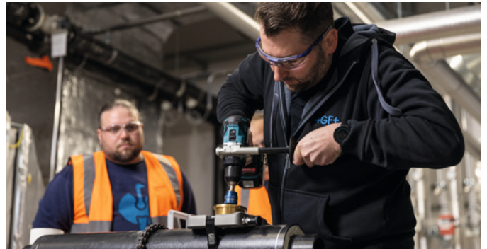
A GF Piping Systems specialist conducted a training course for the installers.
