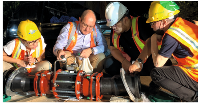
Assembly of piping system and adjusting to the current main line pipe distribution.
