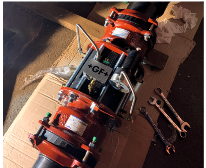
Piping system integrated with NeoFlow DN150 and MULTI/JOINT 3000 Plus at Tangerang, Indonesia.
