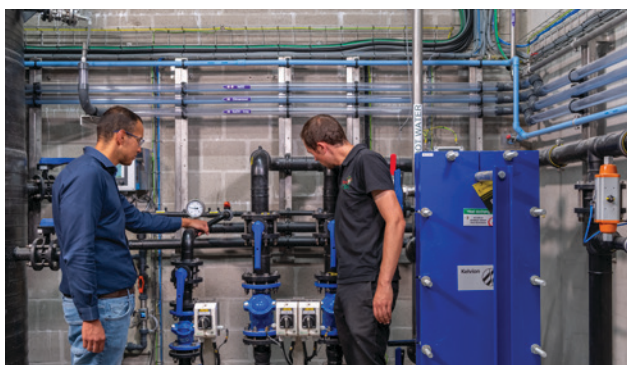
Joeri Tomas Fahim (GF Piping Systems) and Karsten Pauwels (De Halve Maan) at the water treatment plant.
