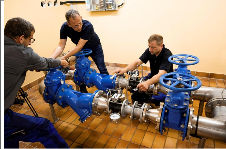
NeoFlow installation in utility network.
