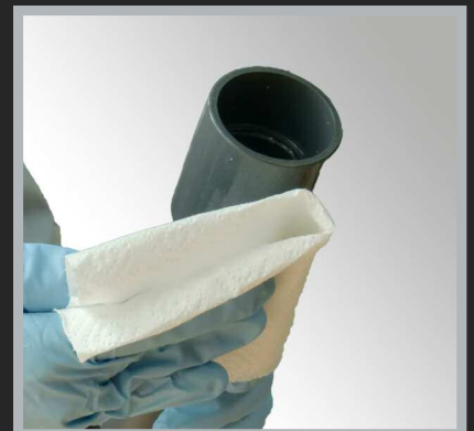
Adhesive bead can be cleaned or be used as a quality proof
