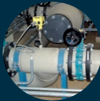
Flue Gas Desulfurization
