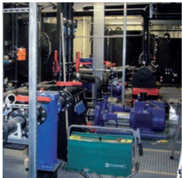
Cooling system for transformers and switch panels.
