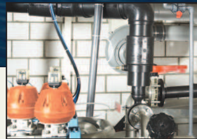
Industrial Wastewater Treatment
