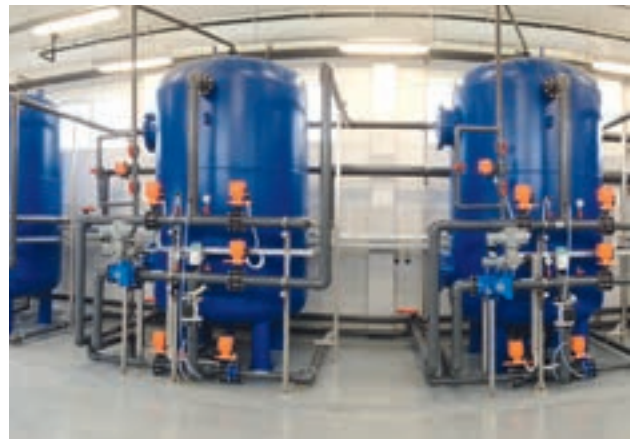
Sandfilter drinking water plant, Virovitica, Croatia.
