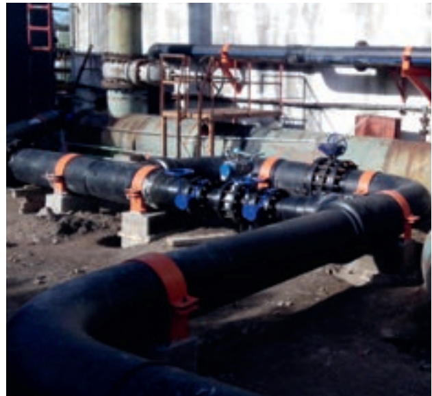
Thermal production processes in petrochemical plants, South America
