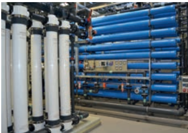
Process water plant, petrochemical industry, Germany.
