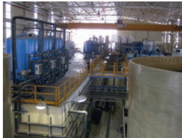
ZLD plant for aluminium coiling company in Greece.
