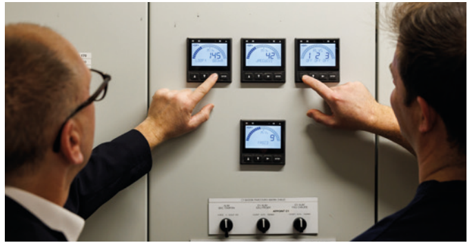
Transmitters such as the 9900 allow the Sofitel Quiberon to ensure the correct water flow in various applications.
