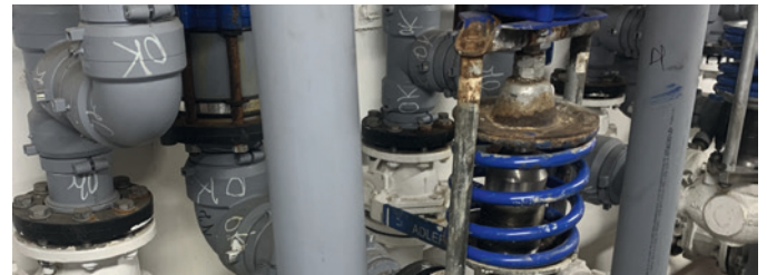
Corroded metal manifold before exchange (provided by MecShip/CCL).
