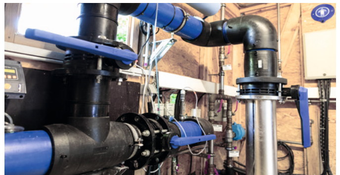
New Butterfly Valve 565 in the filter system
