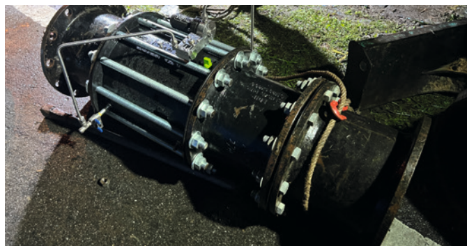
In order to meet the requirement, a DN300 valve was installed, which is 10 times lighter than the previous metal PRV.
