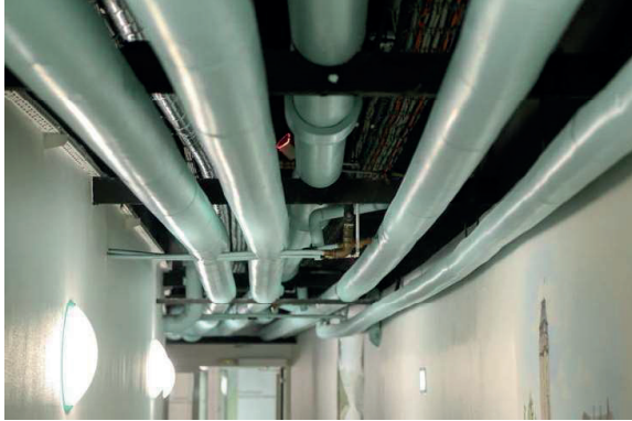
Five different widely-branched pipe systems wind their way through the building complex. The ideal challenge for the Hycleen Automation System.
