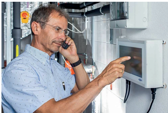
Thanks to the installation, any irregularities which may occur, such as too low temperatures or defective valves and sensors, can now be monitored.
