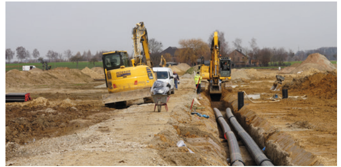
In the "Neuer Soester Norden" development area, pipes are being laid that will later transport the heat from the ground to the 600 residential units.
